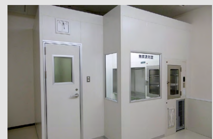
A sterile dispensing room installed at Koto Pharmacy
